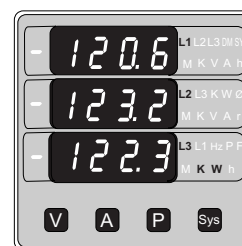
Screen 1 : Phase Active power
